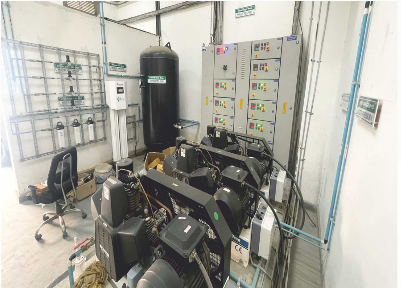
Medical Air Plant
